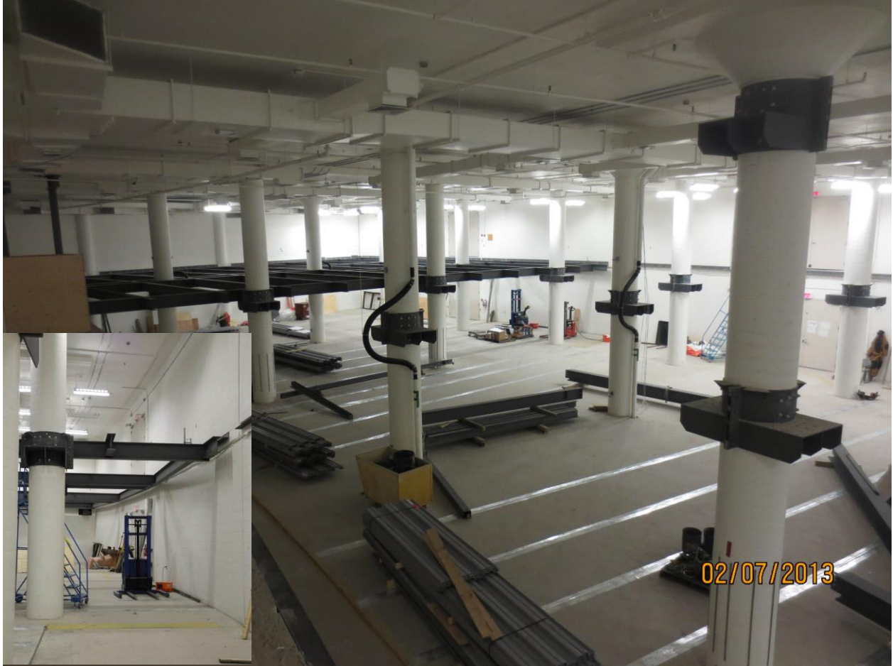
View from 6th floor access of I beams waiting for installation. Installation of I beams shown in inset.
