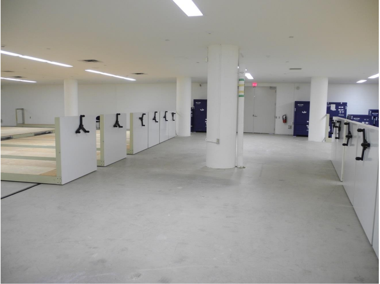
Storage Room 5103 with mobile storage system and lighting installed.
