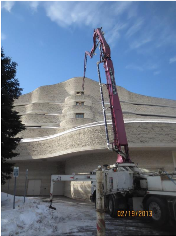
A boom pump delivers concrete to be pumped up 6 floors to pour the structural concrete floor.
