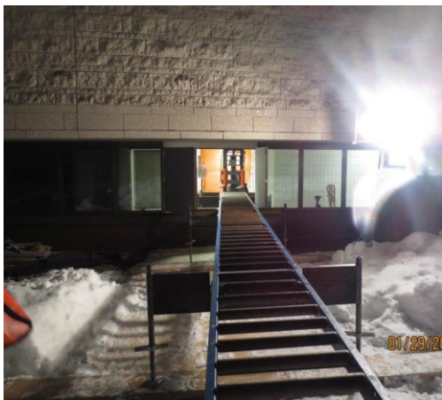
Conveyer system for beam entry.
