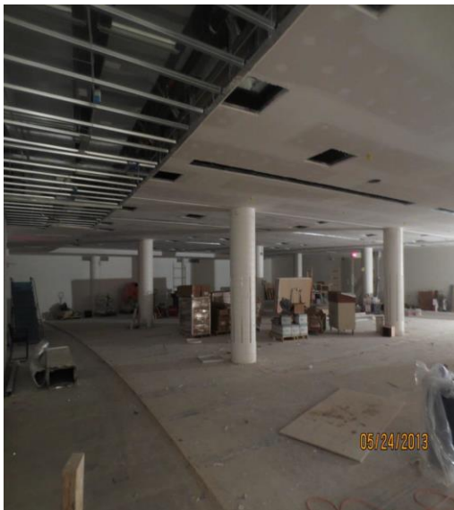
Following installation of the steel I beams, a fireproofing material was applied before a suspended drywall ceiling was added (this image shows the partially installed ceiling).
