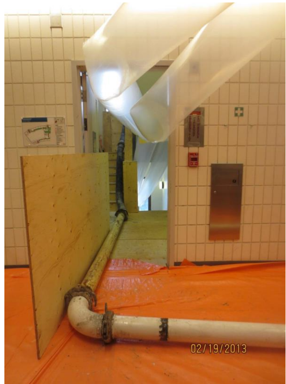
Concrete flows through metal pipes into the 6 th floor storage room. Air ventilation in storage areas was temporarily re-routed via plastic tubing during construction.
