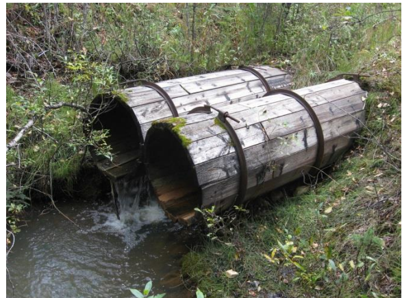
Figure 11. Historic Culverts Site. Two wooden culverts under an abandoned roadway still divert water from a small drainage.
