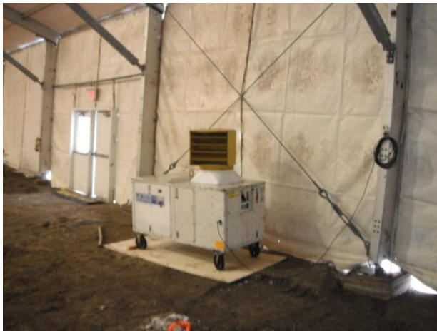
Figure 4. One of four electric ambient heaters inside the tent.
